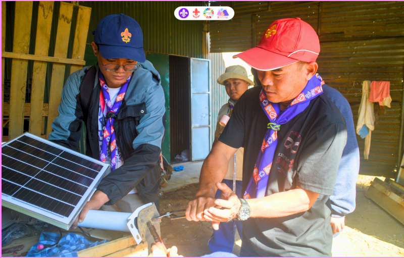
Two Scouts are carefully adjusting the base of a solar-powered light, preparing it to be mounted onto an electric pole.
